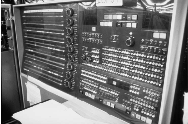
Figure 2. The 1110 was the last system with a full maintenance panel.
