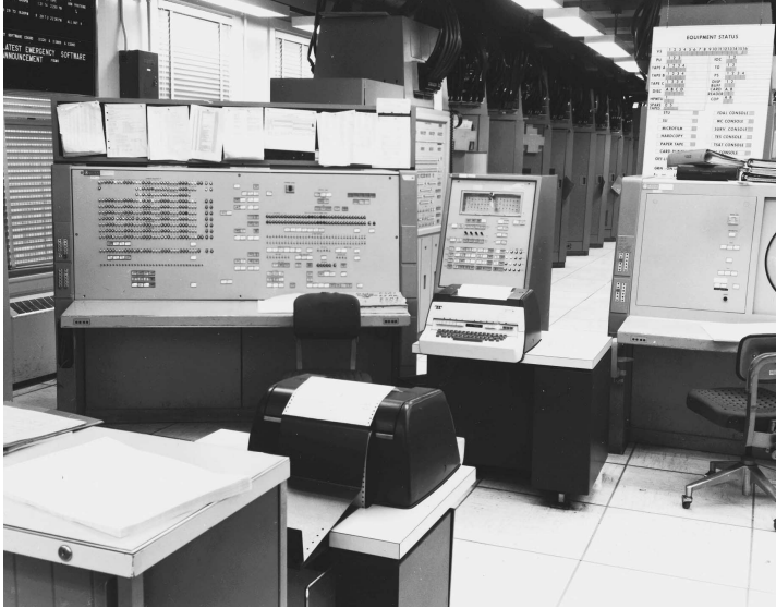
Figure 1. The Nike-X Central Logic and Control module here shows operator control panels in the foreground and a maintenance panel at the back left.
